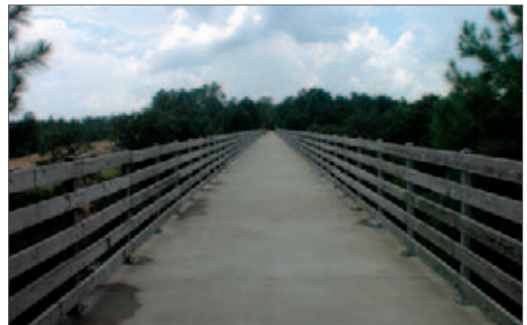
Above: Before and after PATH trail conversion across a rail bridge on the Silver Comet Trail
