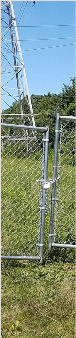
Passive security measures, such as this gate in Nassau County are not common along the right-of-way (ROW). While typically open, many of the entrances to the ROW are overgrown making passage difficult.
