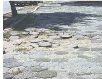
Paved surface with deterioration of hex blocks
