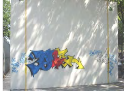
Spray paint on handball court
