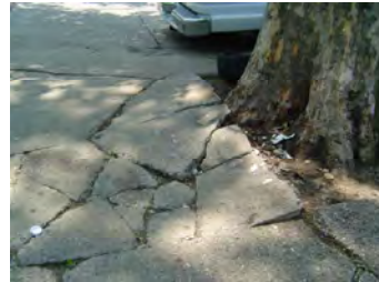
Cracked and uplifted sidewalk
