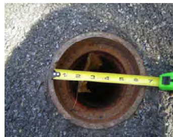
Missing valve cover
