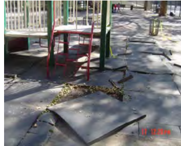
Safety surface damaged in a critical area of the playground
