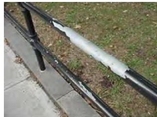
A fence in need of paint
