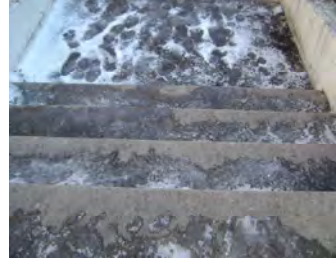
Ice on a staircase, Priority One Immediate Attention
