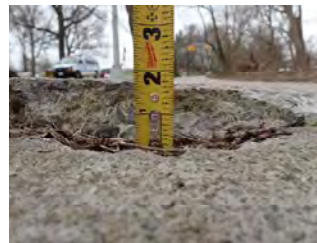
1.5 inch trip hazard
