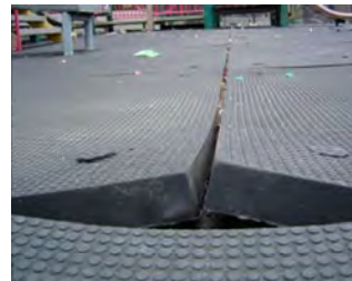
Safety surface uplifted causing trip hazard
