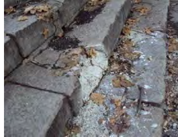
Fall hazard on staircase
