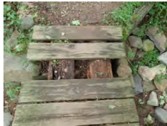
Trip hazard due to damaged footbridge
