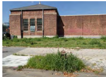
Weeds obscure fire hydrant
