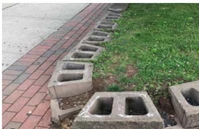
① WALL MISSING CAP
