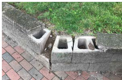
② WALL MISSING CAP
