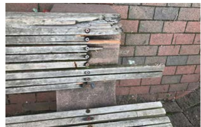
③ DAMAGED BENCH
