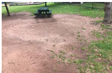
⑤ EVIDENCE OF WATER FLOW
